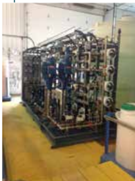
RO system recovers 90% of wastewater stream for Alberta camp
