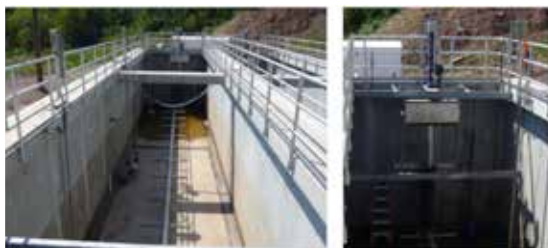
SBR tank with decanter (closeup)
