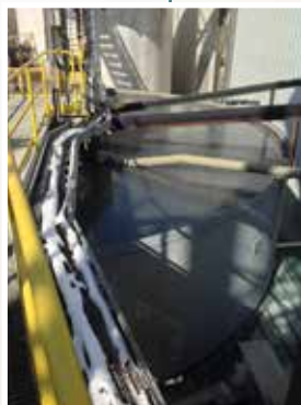
Cyanide destruction process underway in tank
