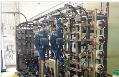
Small RO unit recycles wastewater at a remote oil & gas camp, saving a half million dollars a year in wastewater disposal
