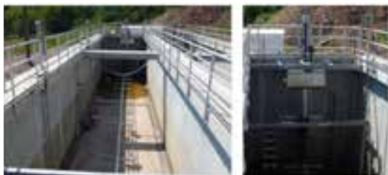
SBR tank with decanter (closeup)
