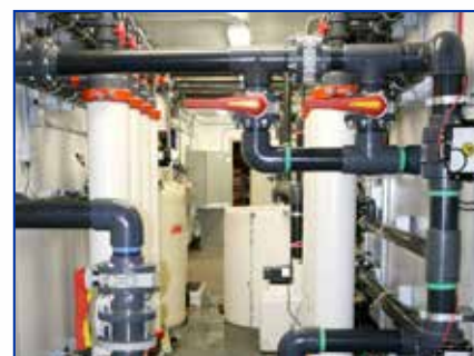
Potable water treatment for potash mine site filters groundwater high in particulates
