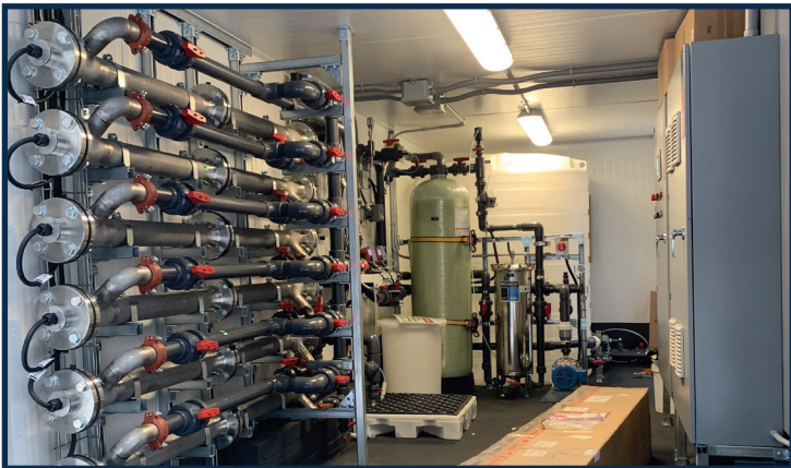
Figure 2: Interior of completed system
