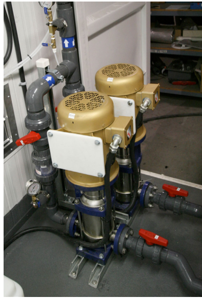
Dual booster pumps
