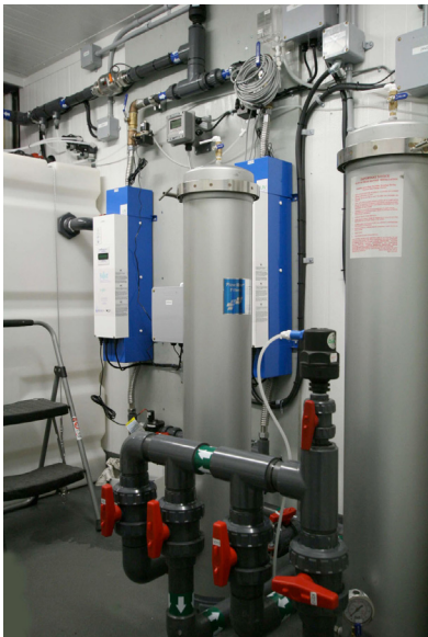
Dual ultraviolet disinfection units
