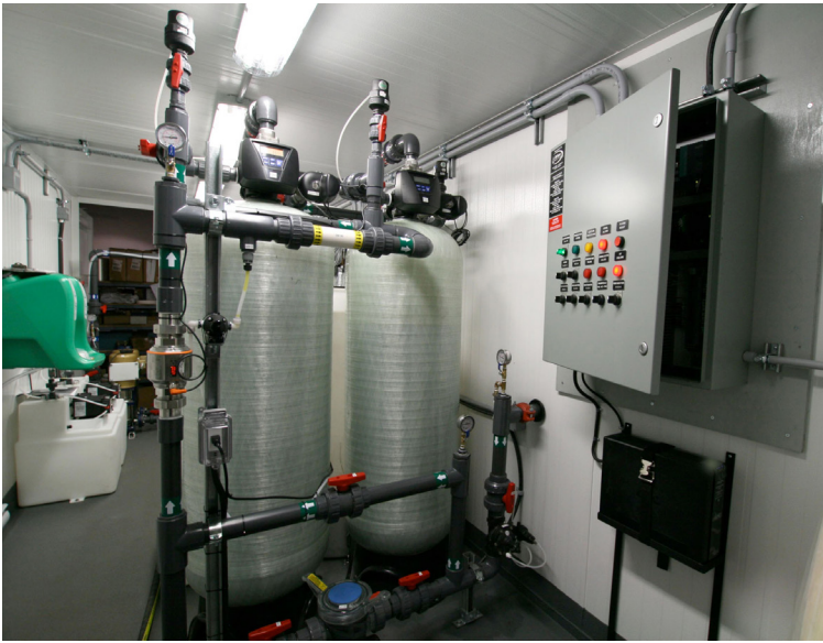
A view of the chlorination system (left), media filters and control panel
