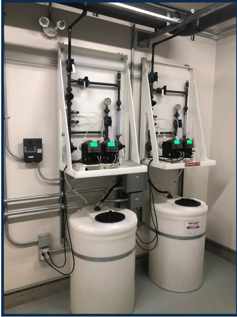
Figure 3: Dual Chlorination system
