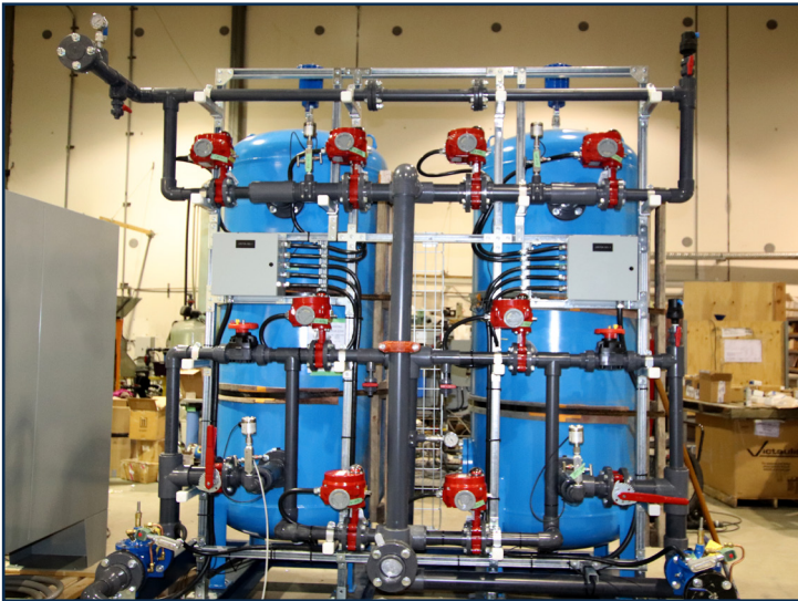
Figure 2: Greensand system on skids
