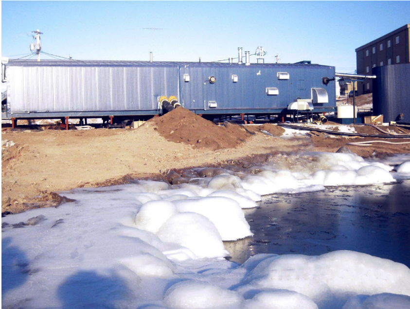
The water treatment plant and backwash tank viewed from the lake. Dual intake lines are shown at center
