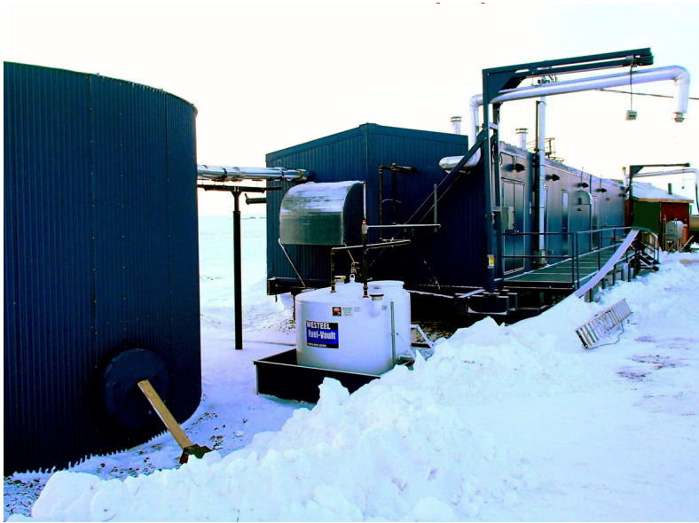
North side view of the water treatment building, truckfill arms and backwash tank during winter operation
