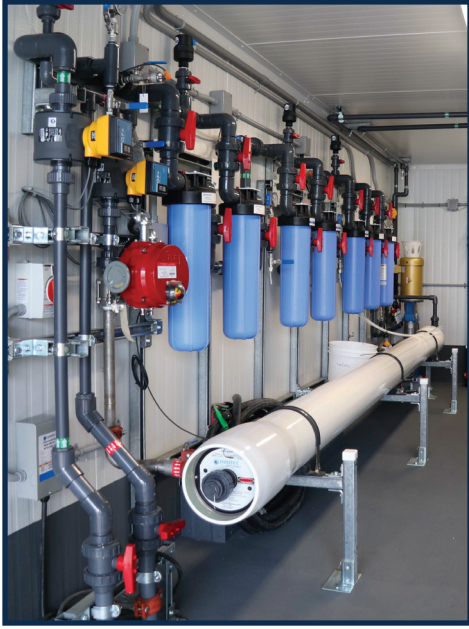
Figure 3: Ultrafiltration skid at UBC
