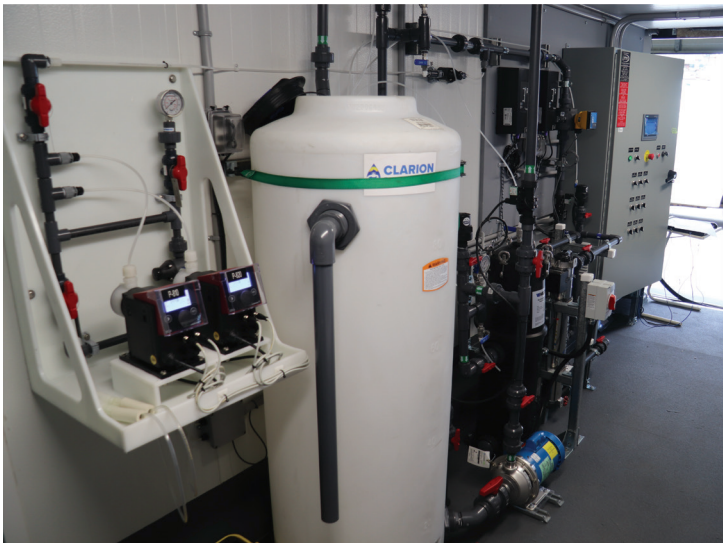
Figure 2: Interior of completed system
