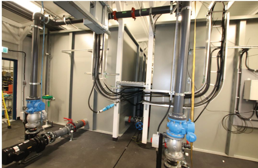
Fig. 8 - Dual 60 cubic meter MBBR tanks housed within modular buildings
