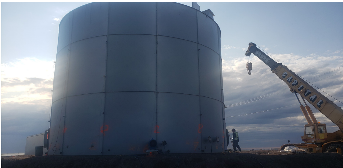
Fig. 3 - Site erection and welding of a large potable water tank for Cambridge Bay, Nunavut.
