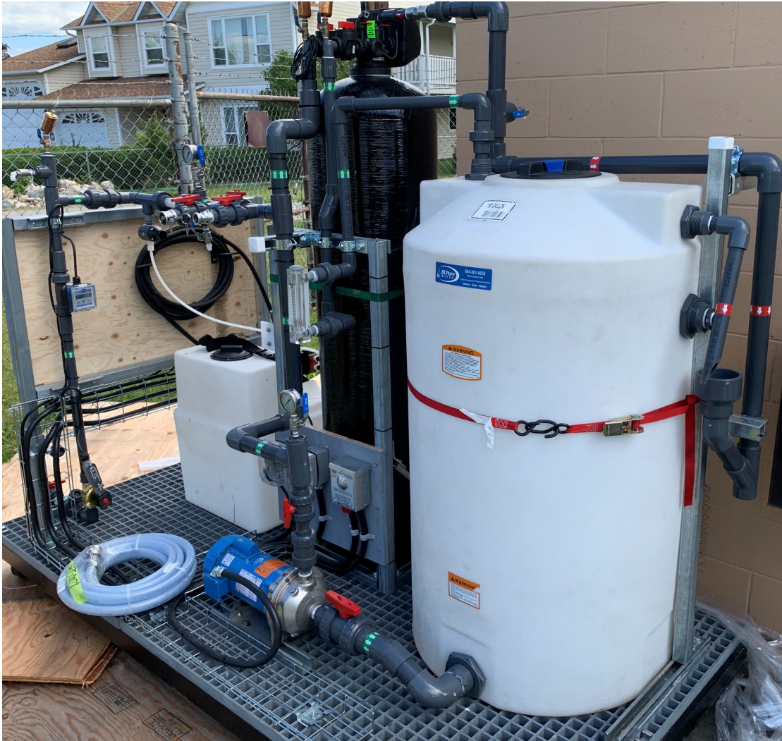
Figure 1 – Backside of the pilot plant showing the backwash tank and pump
