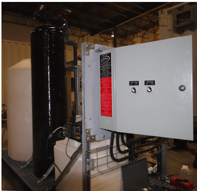
Figure 2 – Frontside of the pilot plant showing the control panel, chlorination system and media vessel
