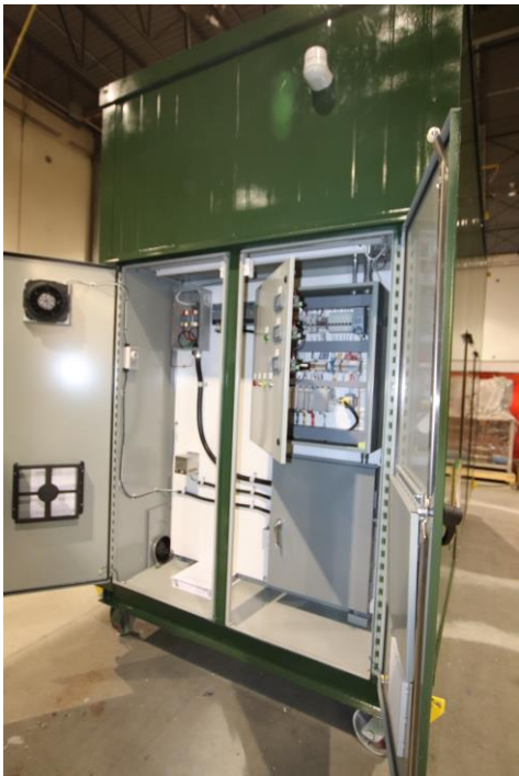
Figure 2 – Electrical Compartment of Kiosk
