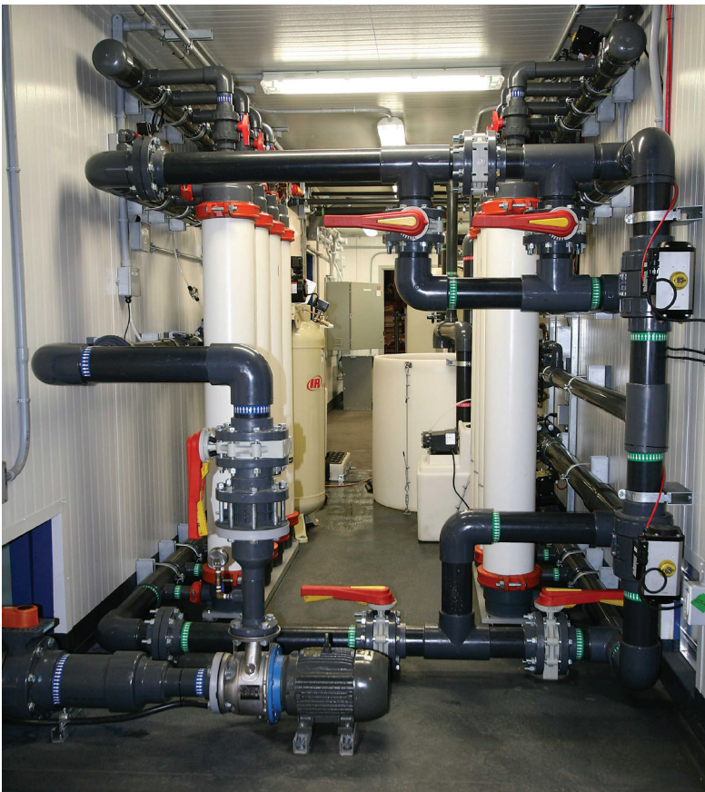
The package water treatment system has ultrafiltration membranes before the RO.
