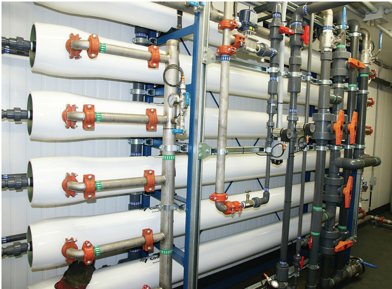
View of the reverse osmosis system with high pressure stainless steel lines.
