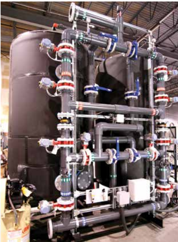
Dual insulated media vessels with a control valve nest
