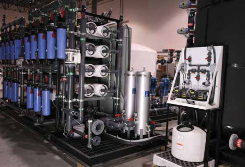
Eight reverse osmosis membranes reduce the level of undesirable contaminants in the water.
