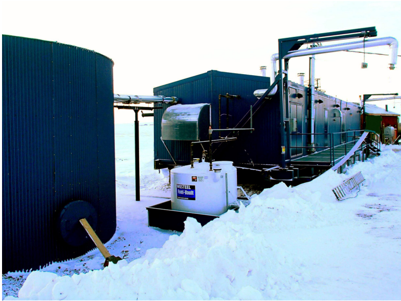
North side view of the water treatment building, truckfill arms and backwash tank during winter operation
