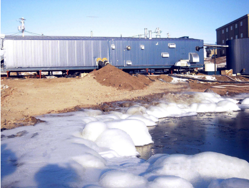
The water treatment plant and backwash tank viewed from the lake. Dual intake lines are shown at center
