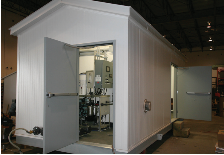
The 10 x 22 foot insulated panel building muffles the sound of the operating generator
