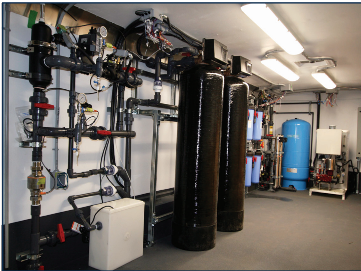
Figure 2: Interior of completed system
