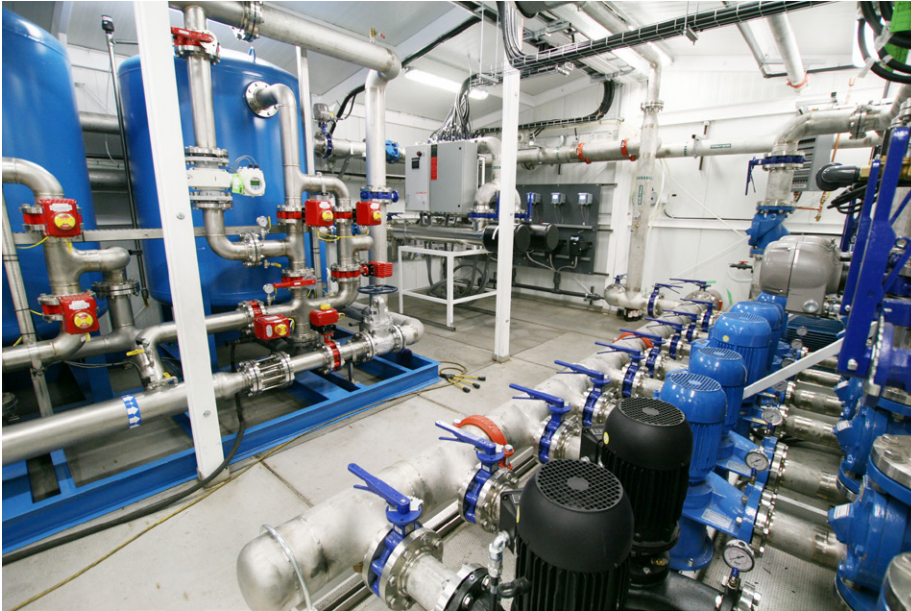
Left to right: The three automatic 48-ft 3 zeolite filters for reducing turbidity, two UV units, turbidity meters, and the major pumps in the main room of the treatment plant.
