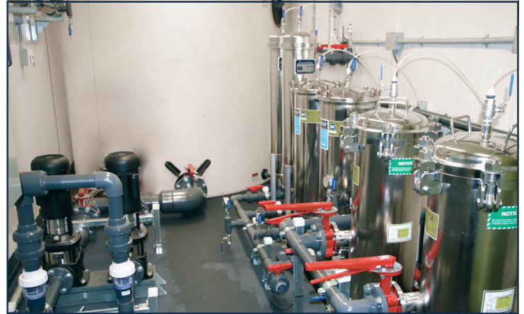
Figure 2: Interior of completed system
