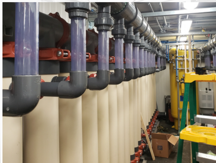
NX Hollow Fiber dNF Membrane Train installed and connected on site.
