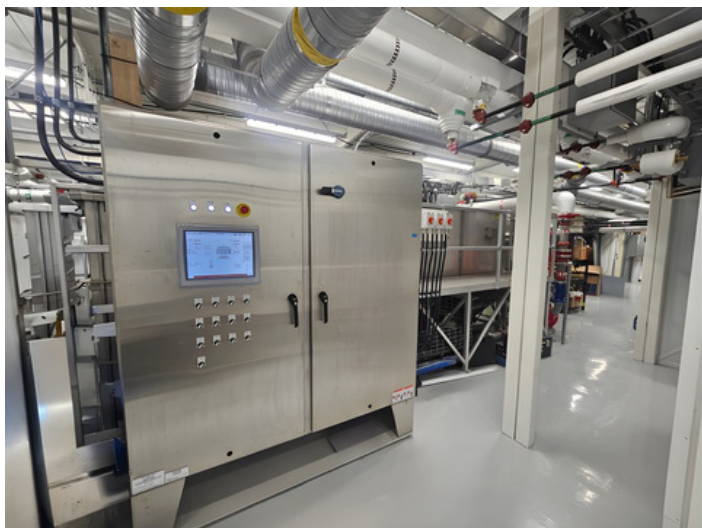
Inside of the Water Treatment Plant
