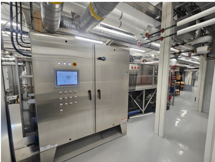
Inside of the Water Treatment Plant
