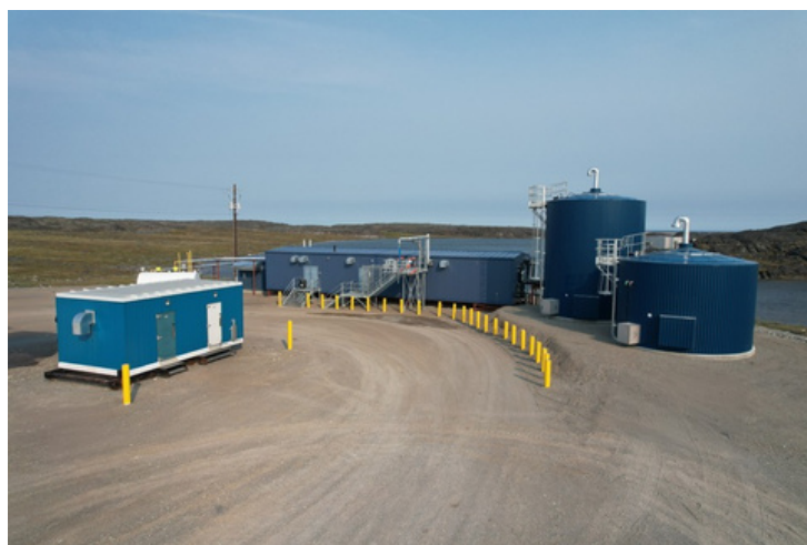
Water Tank and UV - As Delivered
