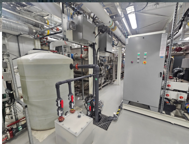
Water Tank and UV - As Delivered
