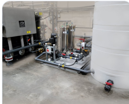
Cartridge filtration and reuse pumping: the last stop before water heads back to the wash bay.
